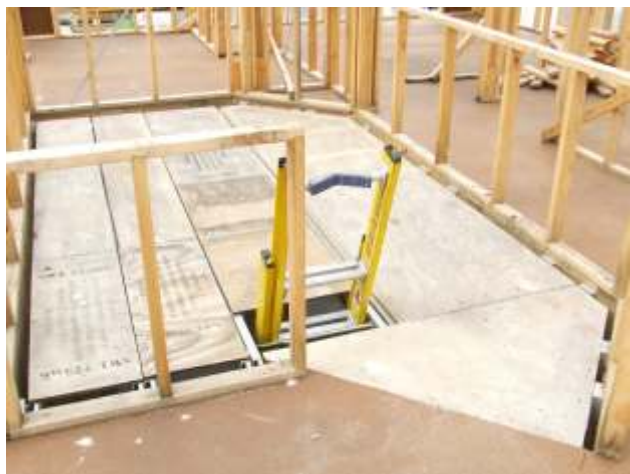
Enclosing a void saves lives.
